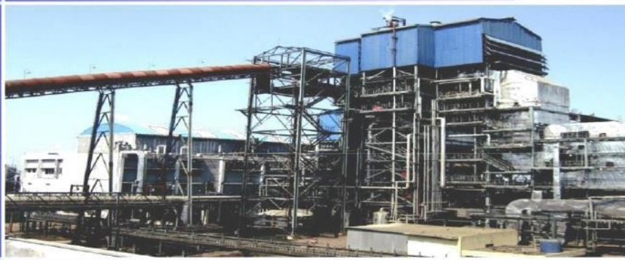
34 MW COGENERATION PLANT IN MUMIAS SUGAR COMPANY BY AVANT GARDE
